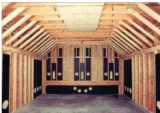
This CAT project, installed 20 years ago, displays the placement of the system’s front stage delivery subwoofers (FSDS) and the dedicated channel subwoofers (DCS).
